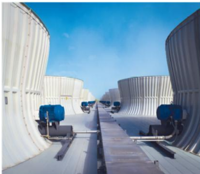
Iatan 2 cooling tower fans. The use of a cooling tower for condenser cooling is an integral part of Iatan's environmentally friendly zero liquid discharge operation.
